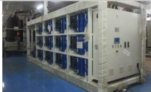
400 MWh VRFB from Pu Neng in Hubei
